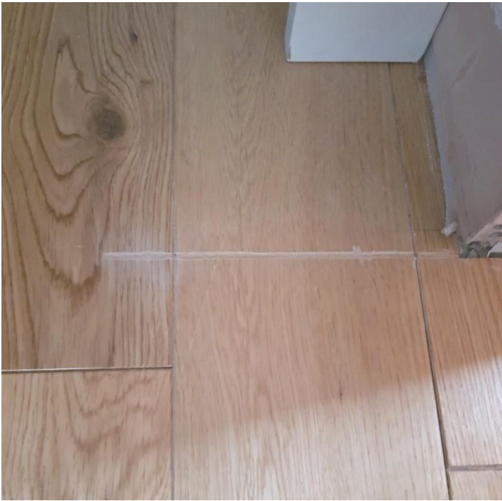
Floor accidentally cut by builders
